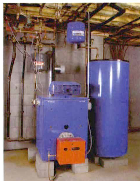
The heart of a hydronic system. This boiler setup provides domestic hot water, hot-water baseboard heat and warm water for radiant floors.
